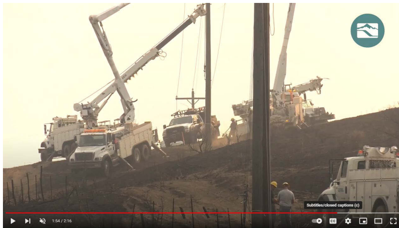
Figure 24 Idaho Power developed an educational video on how we protect wooden poles from wildfire
